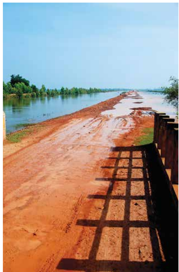
Flooded road to Trapeang Thma dam, Pnom Srok district, Banteay MenaChey (Photo Humanitarian Response Forum 2013)
